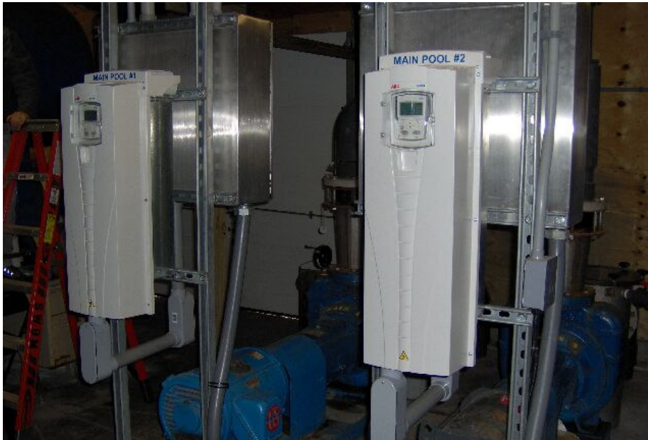
ABB drives added to operate varying pumping requirements of pools at Windsor, CT.
