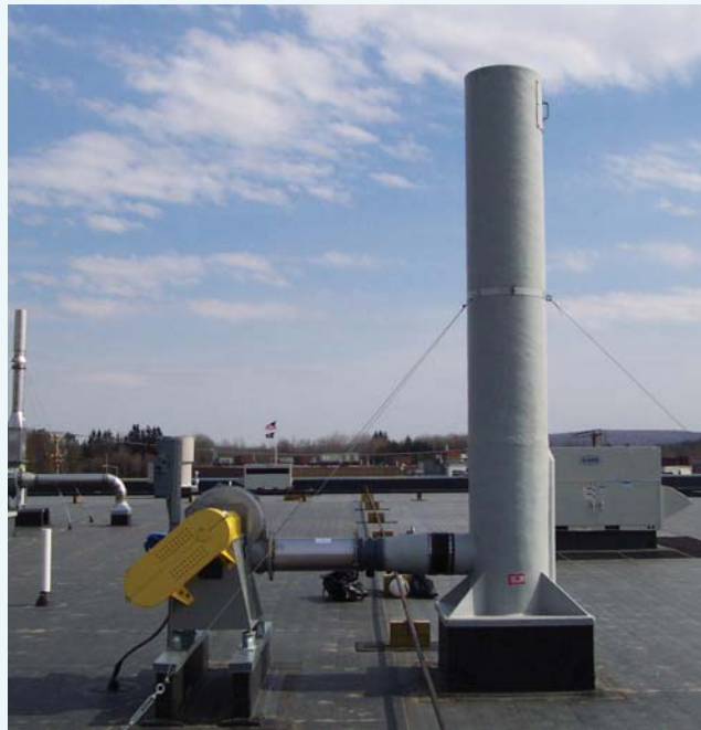
MVT Fiberglass Perchloric Acid Exhaust (Bearing Repair Facility)
