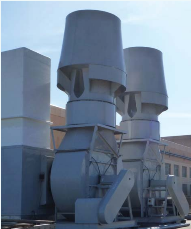
Axijet 6000 Fiberglass High Plume Fans (Wastewater Treatment Plant)
