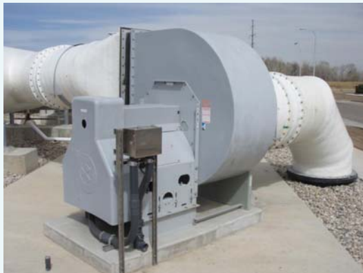
DHK Fiberglass Fan & Fiberglass Ducting at a Wastewater Treatment Facility Plant
