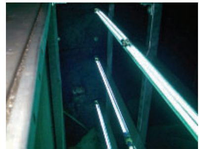
UVC Emitters at COS use germicidal ultraviolet energy to improve IAQ.
