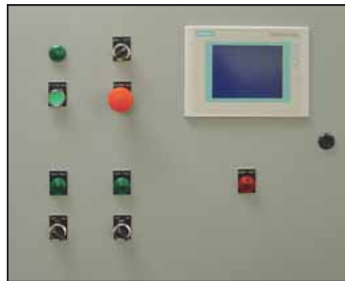
PLC CONTROL PANEL UNIT
